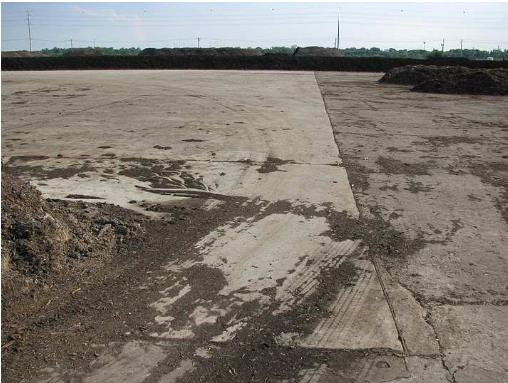
Different view of same concrete composting pad. There should be about a 1% slope on the pad, draining to stormwater catchment/retention and treatment pond.
